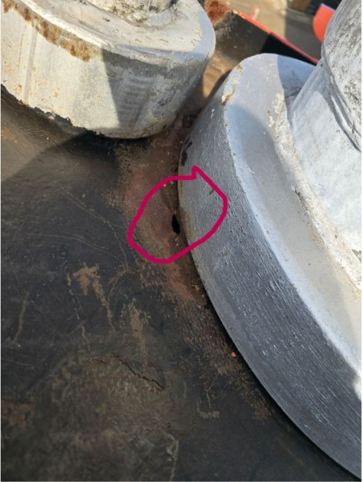
Stbd Exhaust Stack Rain Cap
