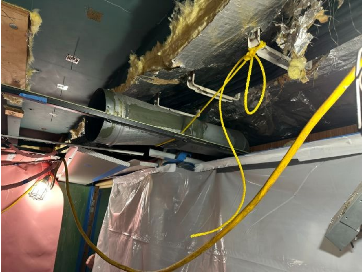
Lounge Overhead Interference
