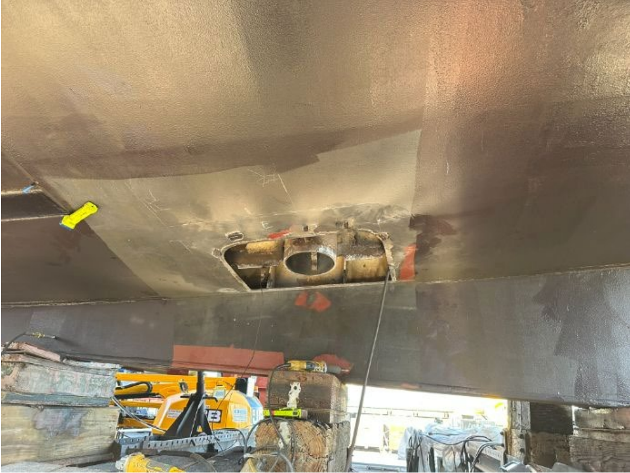
Port Sea Chest- Area of Repair
